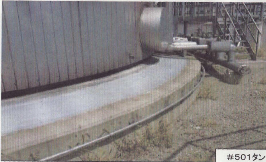
ACT TAPE WH SYSTEM (INSTALLED: 1996)
